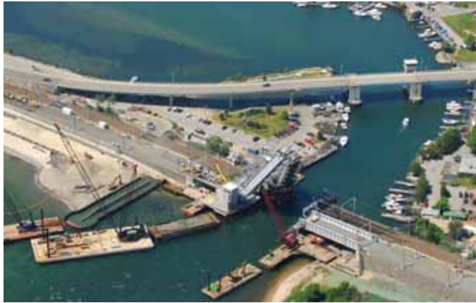
The new Niantic River Bridge at East Lyme, CT, seen June 24, is just upstream (to the left) of the original century-old bridge to its right. U.S. Route 1 is curving in the background.
